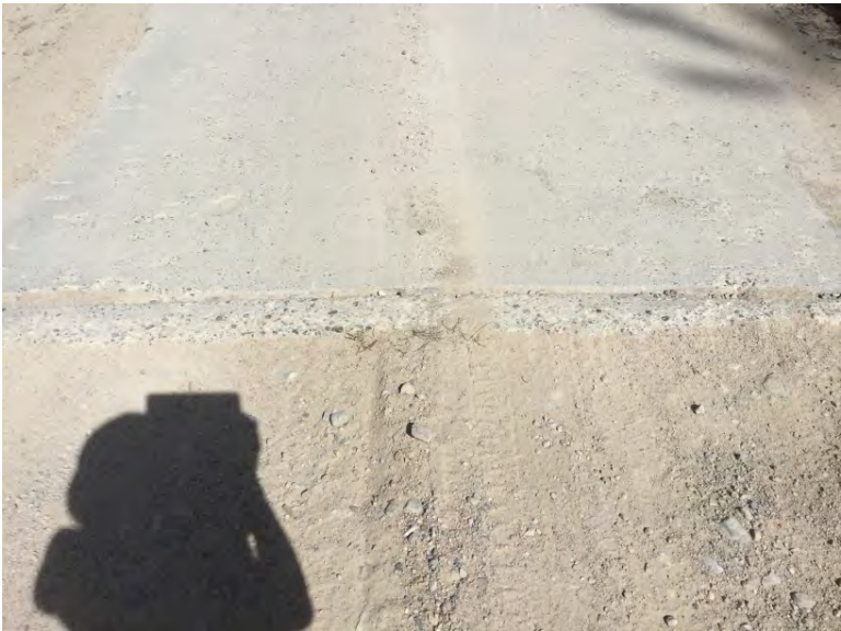
Minor damage to top of ballast wall and panel 1 at right bank
