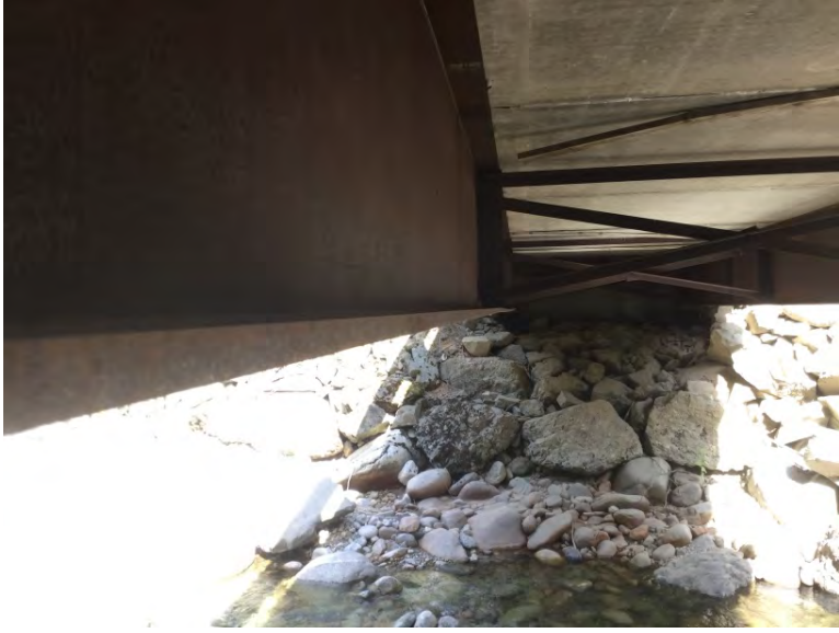
Upstream girder has slight deformation on bottom flange
